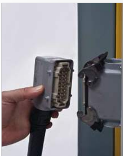
Plug connection to the control panel
